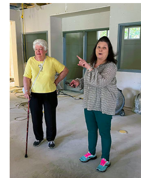
Foundation Board member Jeanne Davis and Branch Manager Lesia Schnur discussing the construction
